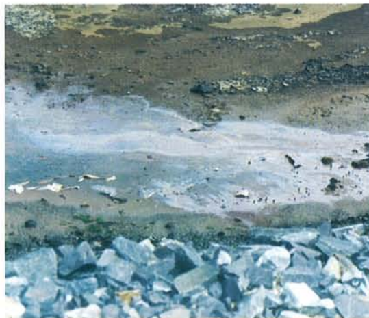
The seepage of hydrocarbons and ground water from a clay embankment.
