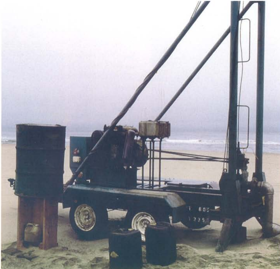
Test pumping rig at the beach at Paaltjies, south of Walvis Bay.
