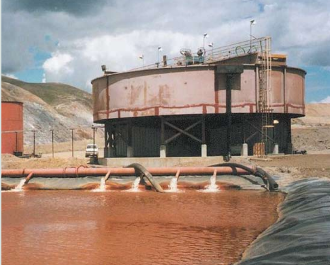
Ferric sulphate arsenic precipitation plant
