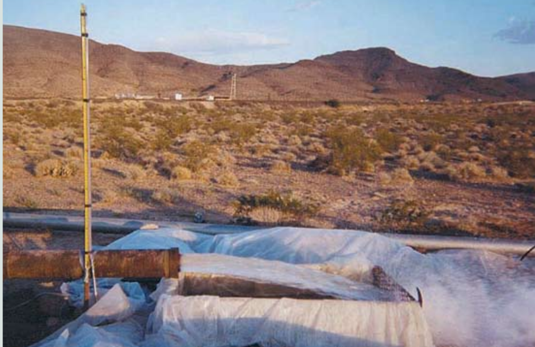
A pressure transducer allows flow rate to be continuously monitored and recorded
