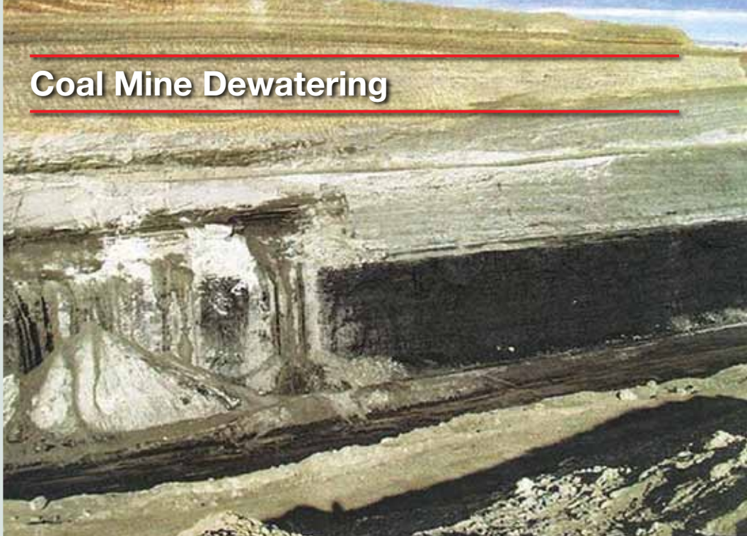
Unstable highwall due to saturated overburden in the Fort Union Fm., Powder River Basin, Wyoming
