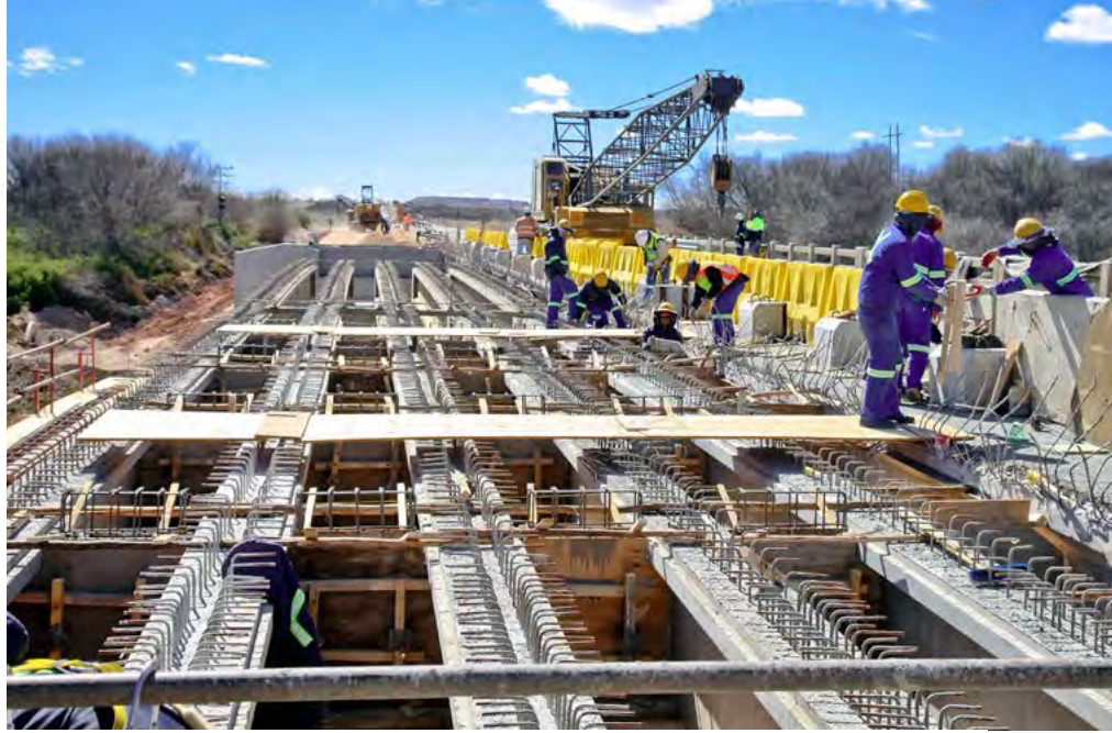
Suppliers of construction materials should be equipped with the relevant expertise, systems and operational capacity to deliver material to increasingly tighter tolerances, consistently and reliably
