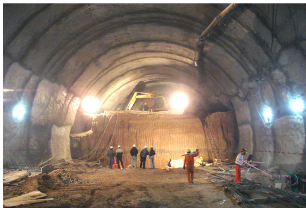
Figure 8. Face view of Case 4, Corrientes Station (Sfriso 2007).
