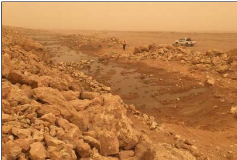
Figure 6: Seepage at the embankment downstream toe.
