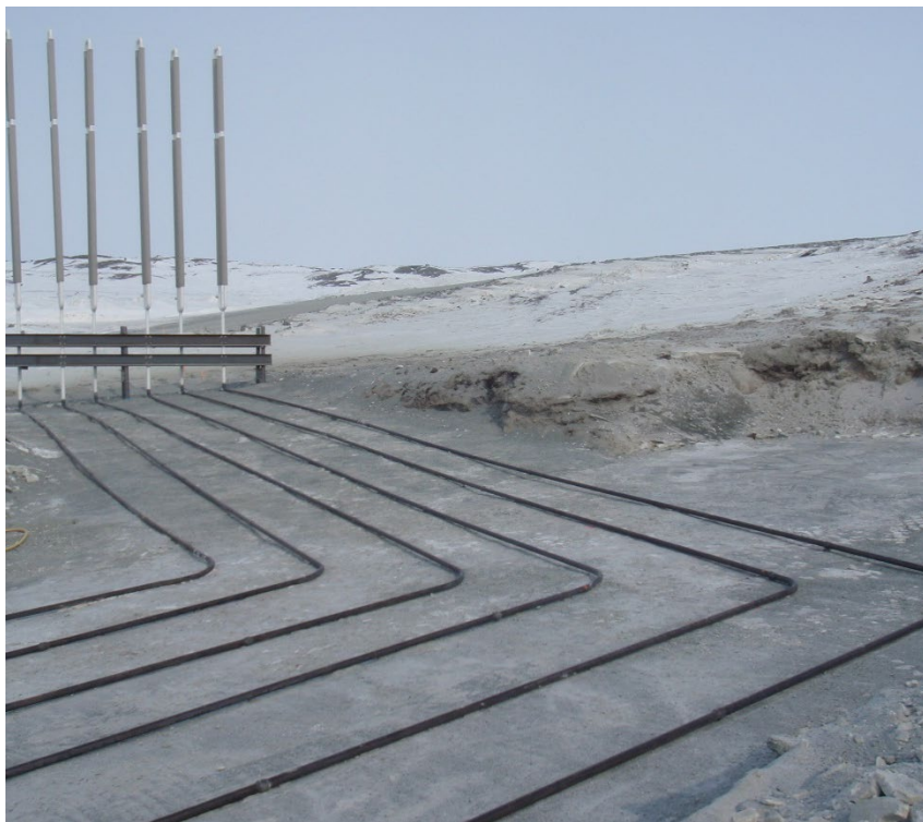
Thermosyphon evaporator pipes connected to radiator
