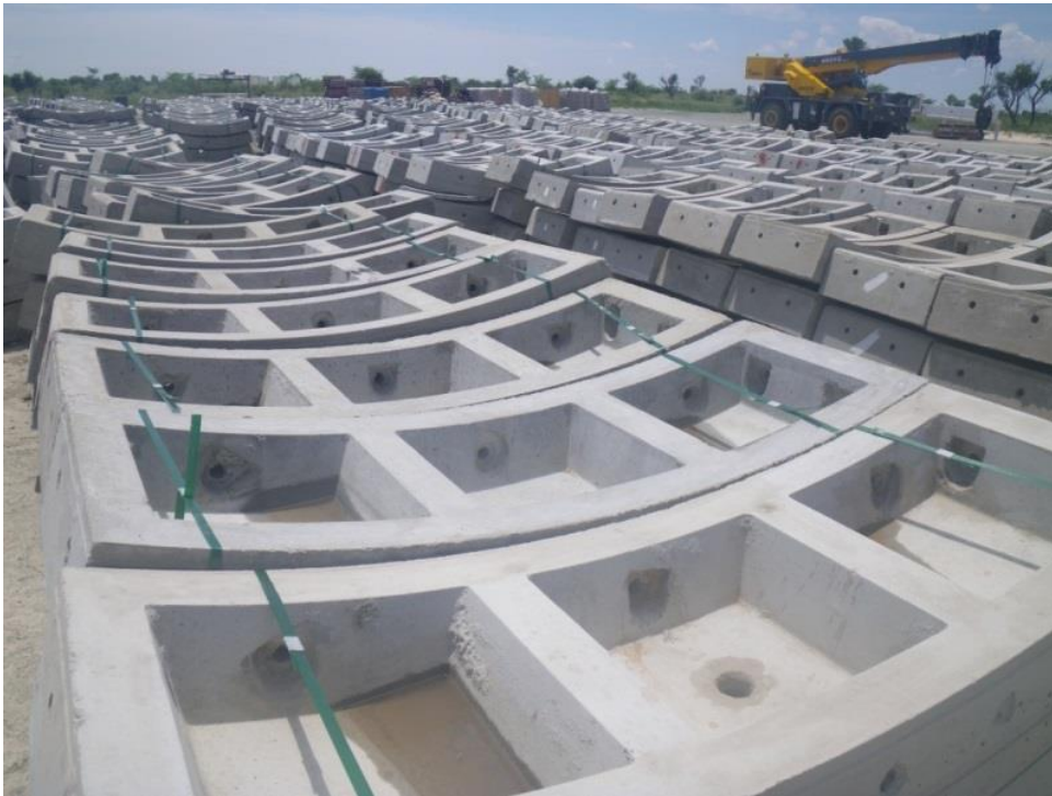
Figure 10: Storage of concrete segments after transportation to site in preparation for underground assembly
