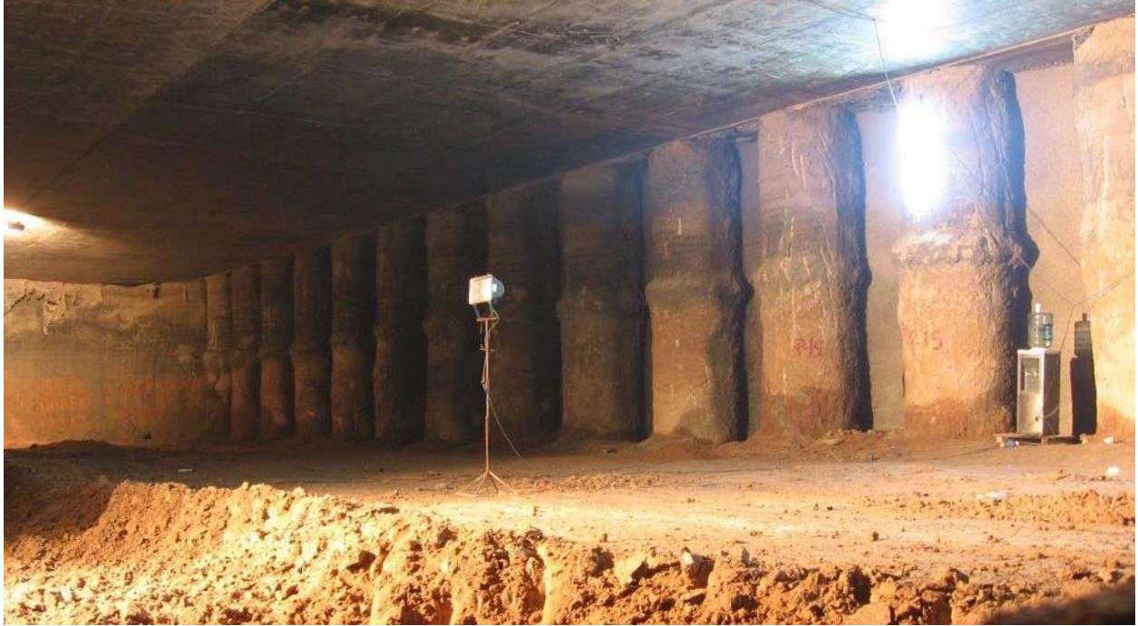
Figure 28. Bulging of piles at the end of the cased portion.
