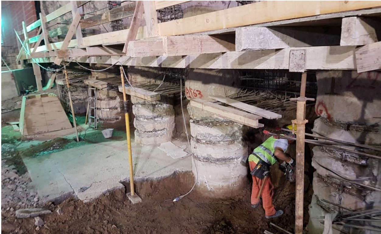
Figure 15. Structural detail of the connection of the invert to the lateral bored piles.
