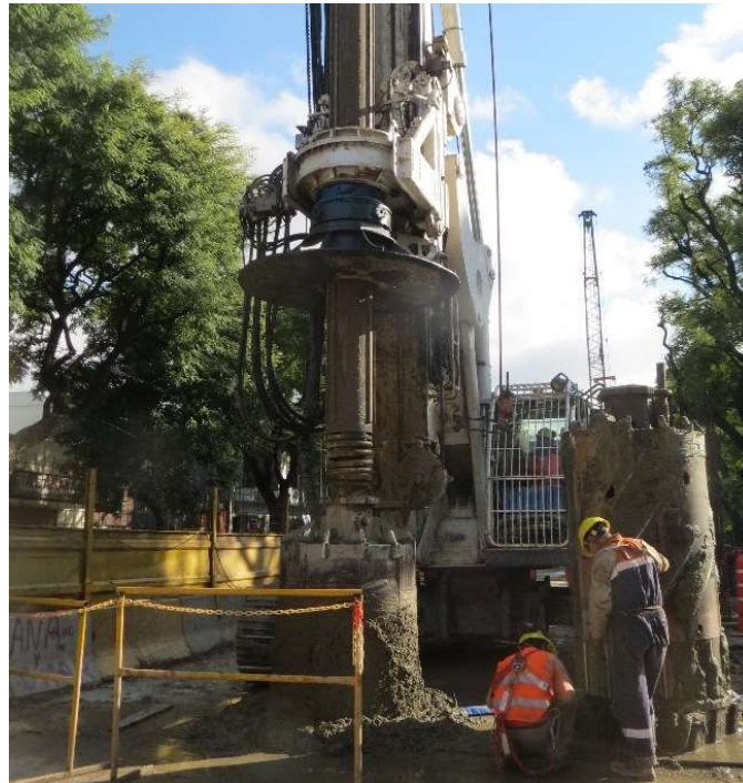
Figure 33. Soilmec SR-70 piling rig provided with two buckets and no casing during the construction of the secant pile wall at Pre-Hospitales tunnel.
