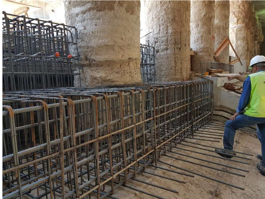
Figure 16. Reinforcement of the slab connected to the (future) wall between the piles.
