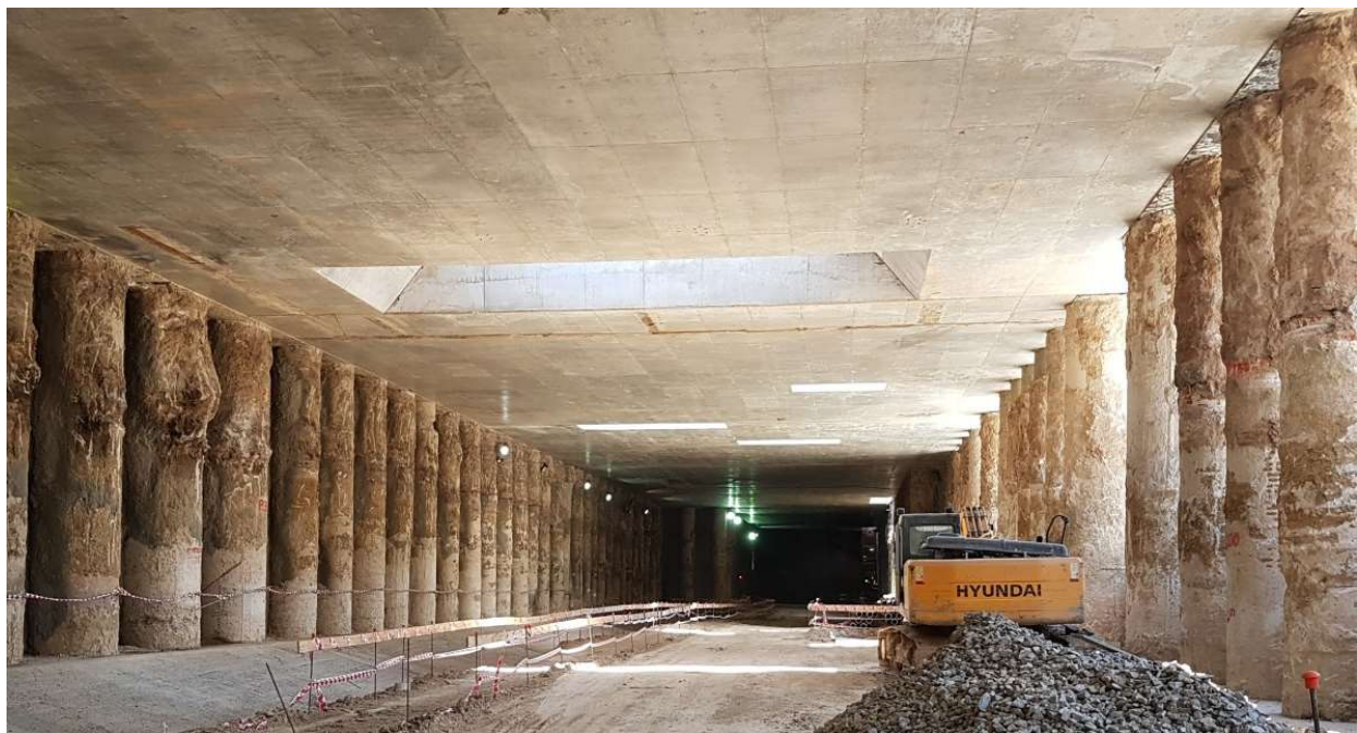
Figure 21. Construction defects in the portion of the bored piles excavated in the man-made fills and superficial soft soils. Note the systematic over-excavations and exposure of reinforcement.
