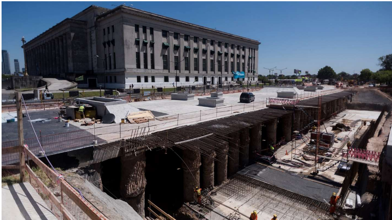
Figure 17. Panoramic view of the underground station during the open-trench excavation of the mezzanine, and the building of the School of Law.
