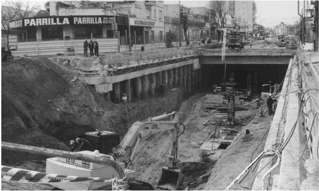
Figure 7. Tronador Station. Note piles with no head support working in cantilever mode.
