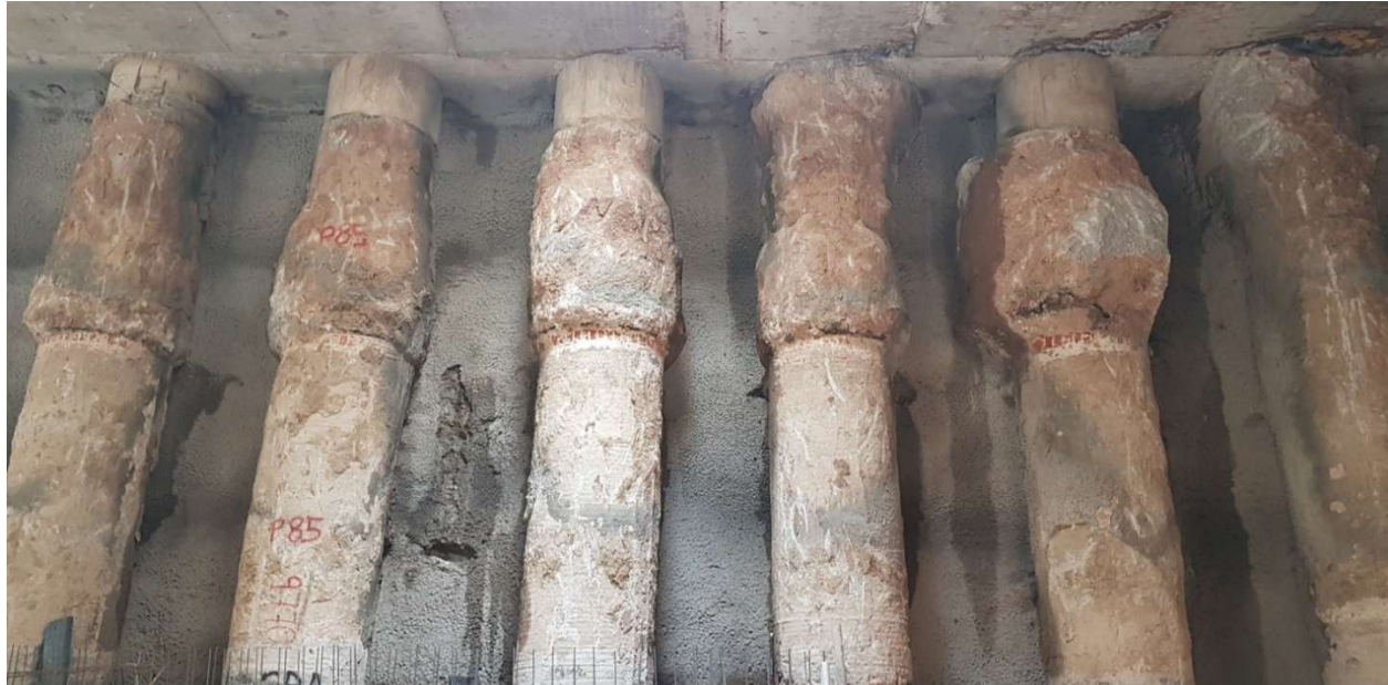
Figure 20. Construction defects in the upper portion of the bored piles.
