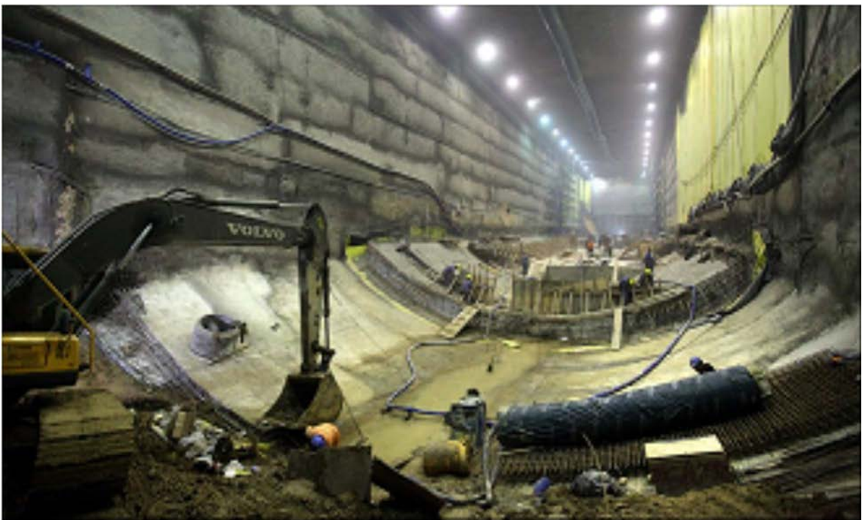
Figure 26. Correo Central Station. All construction stages of the invert including the installation of the geomembrane and the casting of the final invert.
