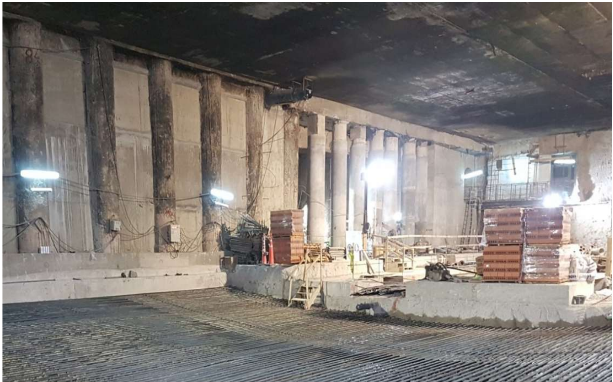
Figure 14. Panoramic view of Line D Maintenance Facility during construction of the invert.
