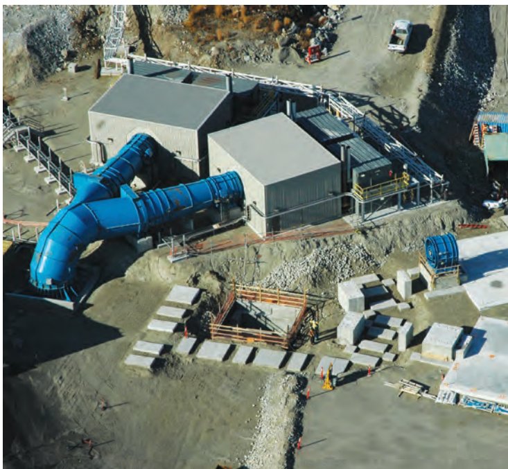
A Stantec twin intake fan and heater installation in Canada
